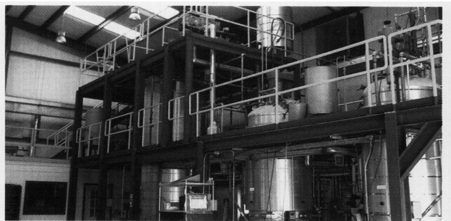
Large-scale TVA facility in Muscle Shoals, Alabama processes biomass feedstocks such as sorted municipal solid waste and agricultural residues into fermentable sugars, which are converted into ethanol.
