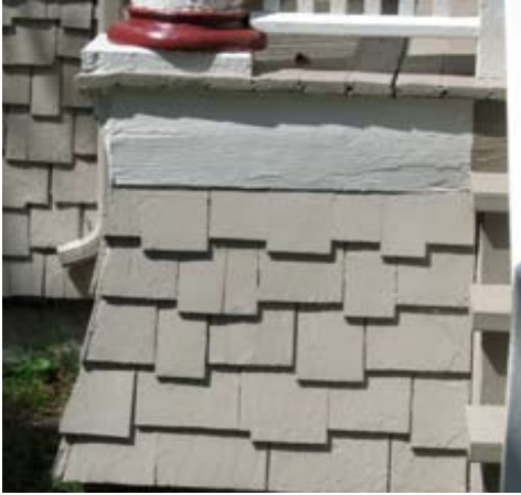
These saw-tooth shingles are a character-defining feature of this home, and should not be replaced with vinyl or other synthetic siding materials.
