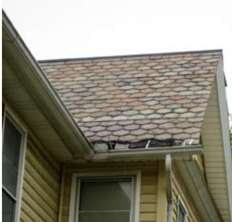
The deteriorated condition of this slate roof will eventually damage the entire roofing system.
