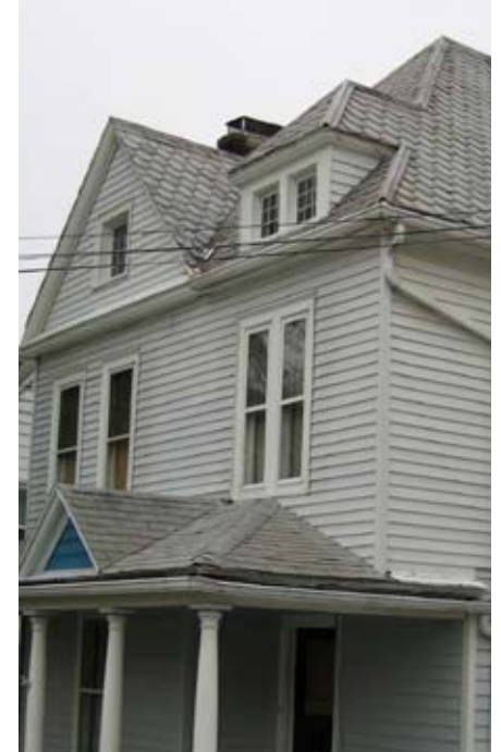
The asphalt shingles on the porch roof should match the original fish-scale slate tiles on the historic roof.
