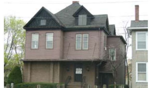
i. Renovations and addtions should not use dissimilar materials, design, fenestration and massing.
