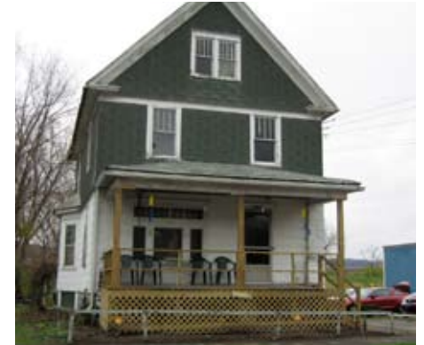
Porch additions or alterations should match the material and design of the original. Modern framing material will alter the character of the entire building.
