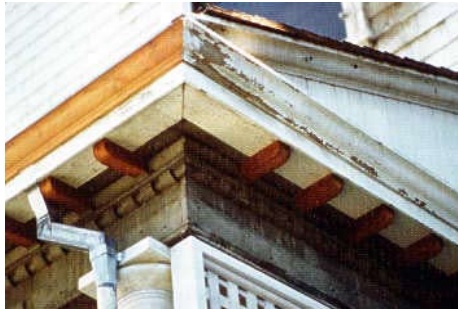
An example of replacement in kind: the damaged portion of this cornice has been replaced, while much of the original has been retained.
