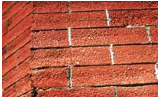
f. Use the gentlest cleaning method possible. Sandblasting will damage masonry.
