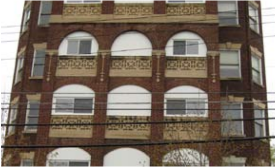
a. Removing historic windows can drastically alter then entire facade.
