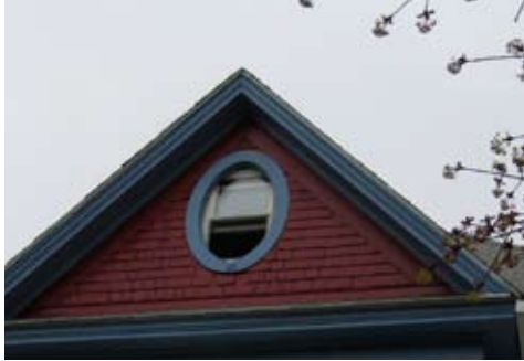
This replacement window does not match the oval shape of the original opening.
