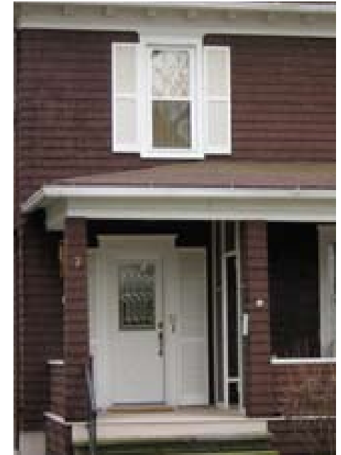
This metal replacement door does not match the materials or character of the rest of the home.
