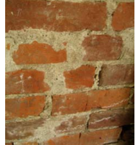
When repointing historic brick, it is important to match original mortar joint profile and composition.
