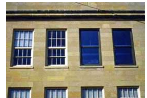
Tinted glazing does not match the historic windows, and is not recommended.
